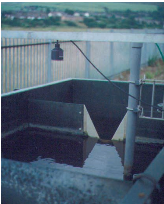
V-Notch Weir Flow Monitoring
