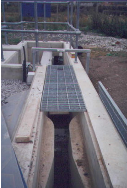
Open channel flow monitoring in a typical flume
